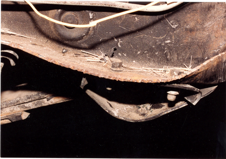
35. Close-up view of the lower flange of the left frame rail in the area adjacent to the CNG tank failure and just forward of the left spring shackle bolt highlighting conversion alteration by retrofit operations
